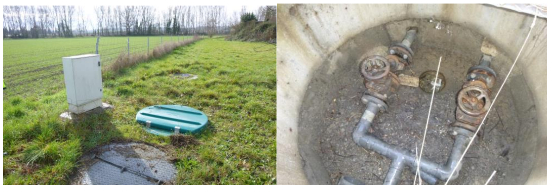
Figure 27 : Equipements corrodés - PR Florallies
