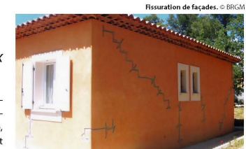
Fissuration de façades. © BRGM
