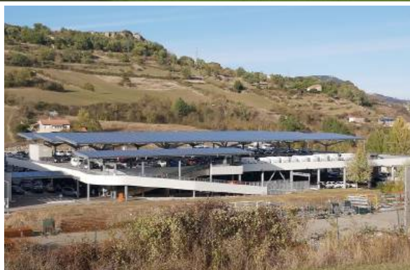
Ombrière de parking, Creissels (12). © Étienne Louyriac
